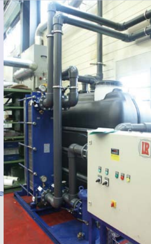
Cooling of lubricating oil for extruding presses.
